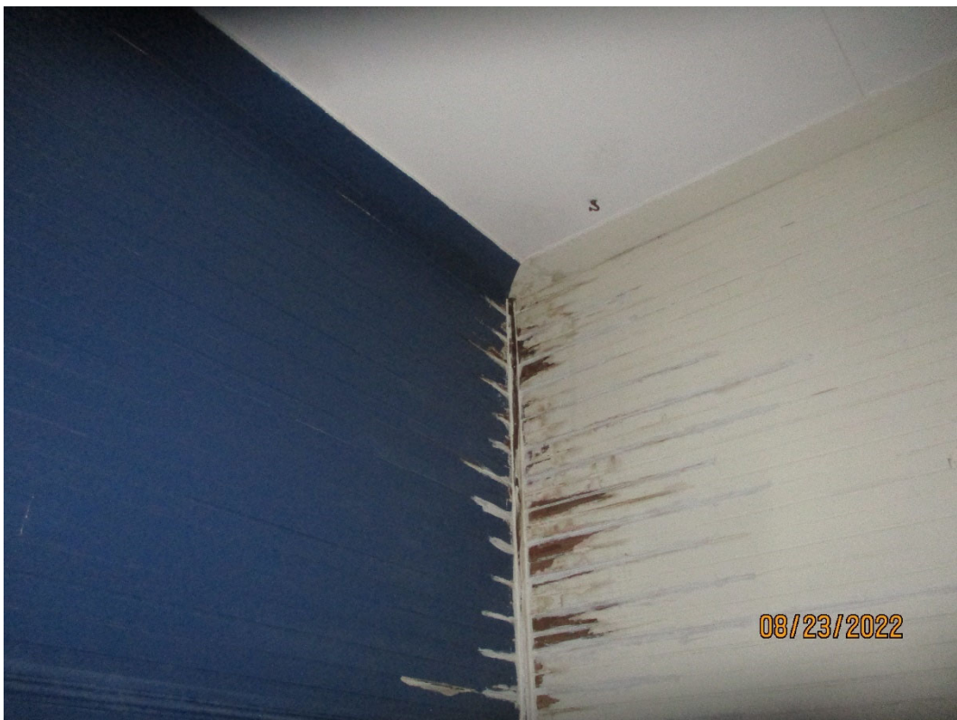
Water damage in main level of original house
