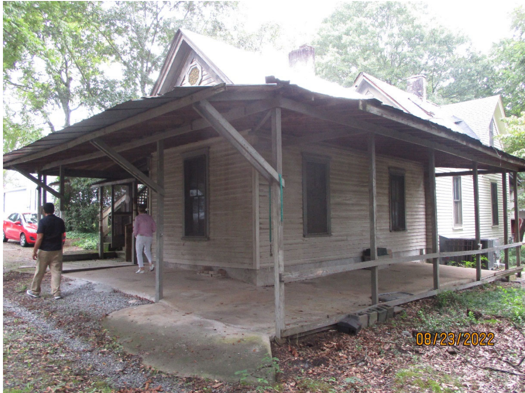
Rear porch is poorly constructed with severely overspanned structural members
