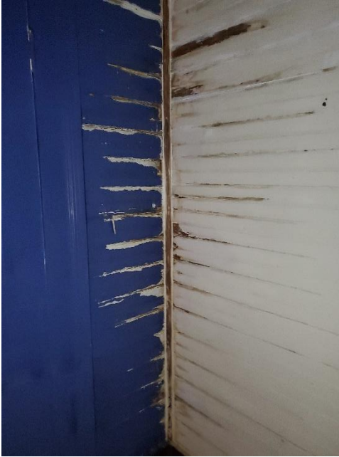
Figure 16 water damage on wood plank walls in dining room corner
