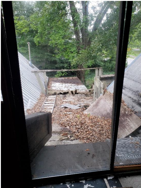
Figure 27 attic deck showing debris build-up and damaged plywood
