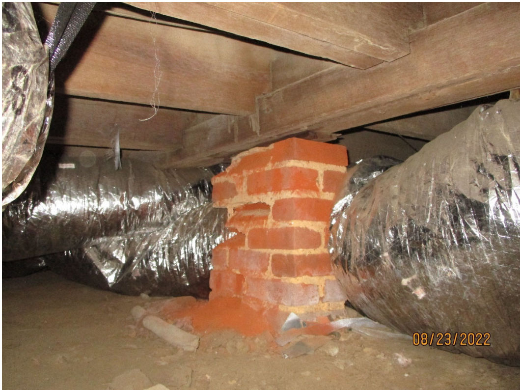
Crumbling foundation(2) support hallway wall
