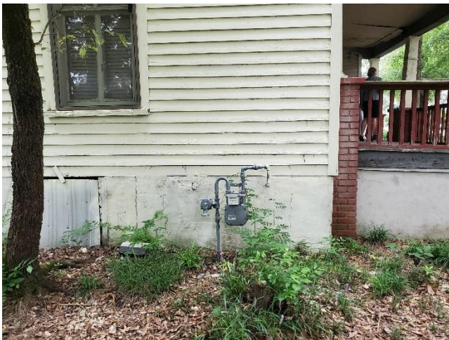
Figure 11 Foundation showing cracking
