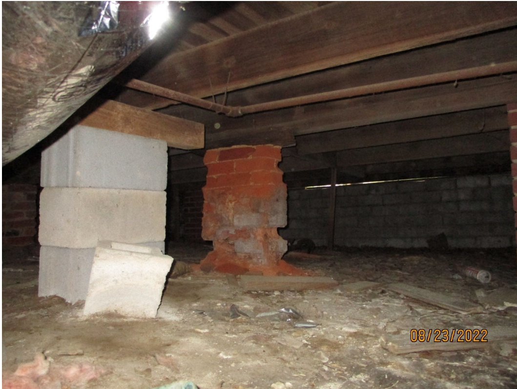
Crumbling foundation(1) supporting front exterior wall
