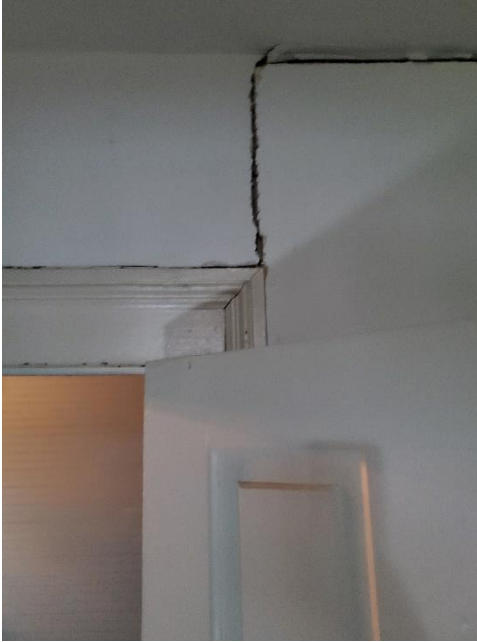
Figure 18 cracking in middle bedroom (bedroom 2)
