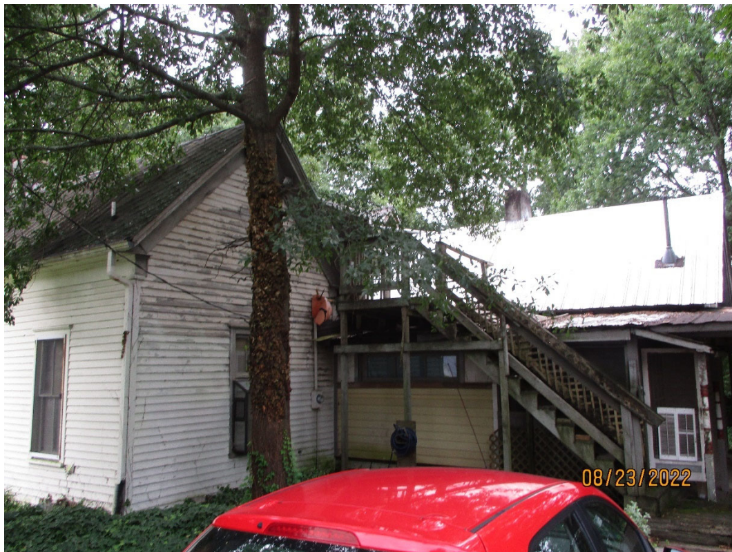
Exterior stair to upper addition is poorly constructed, not accessed for safety concern
