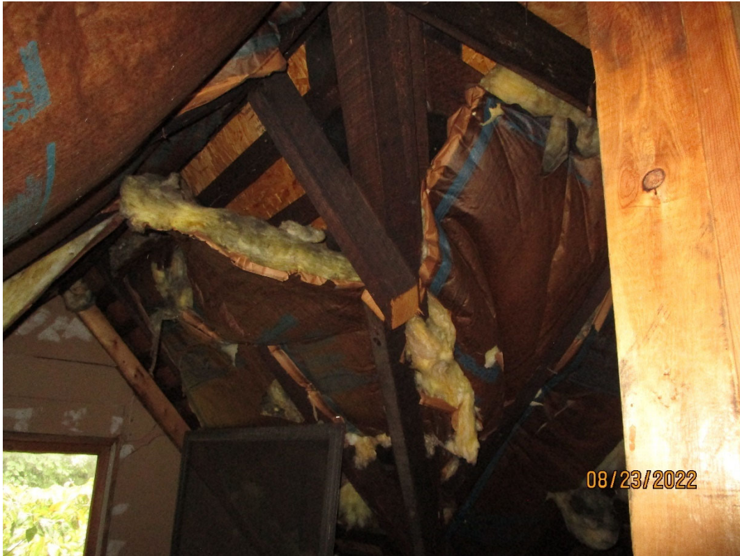
Original roof structure cut with no support to allow hallway access.
