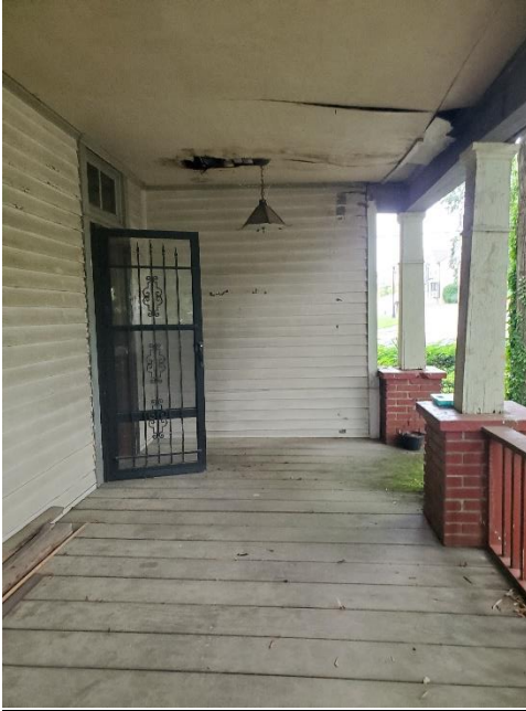
Figure 8 Front porch showing column rot and ceiling damage
