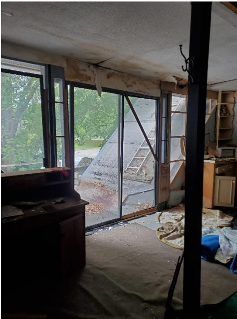
Figure 25 attic living room showing water damage. This damage extends into the hall below.
