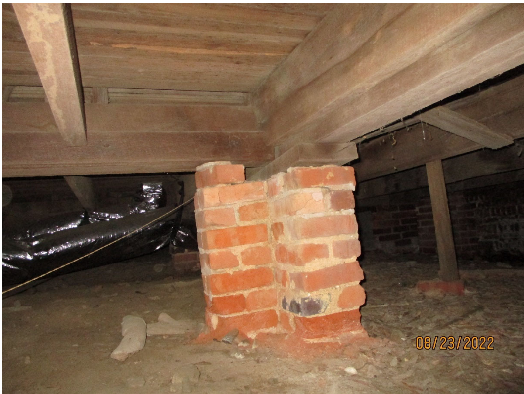
Crumbling Foundation(4) supporting front exterior wall
