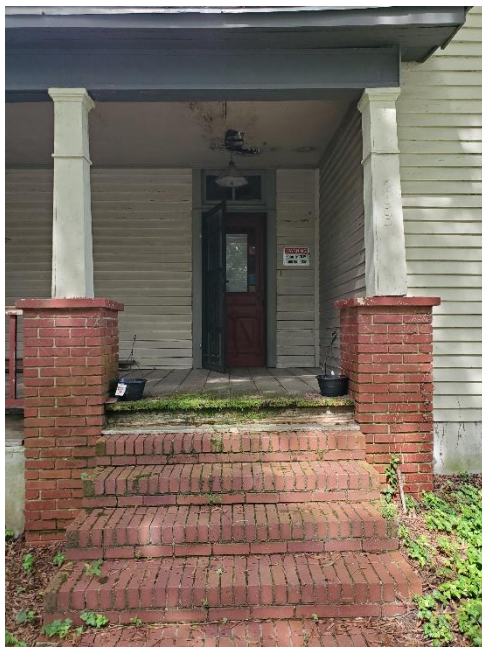
Figure 7 Front steps showing porch and column decay
