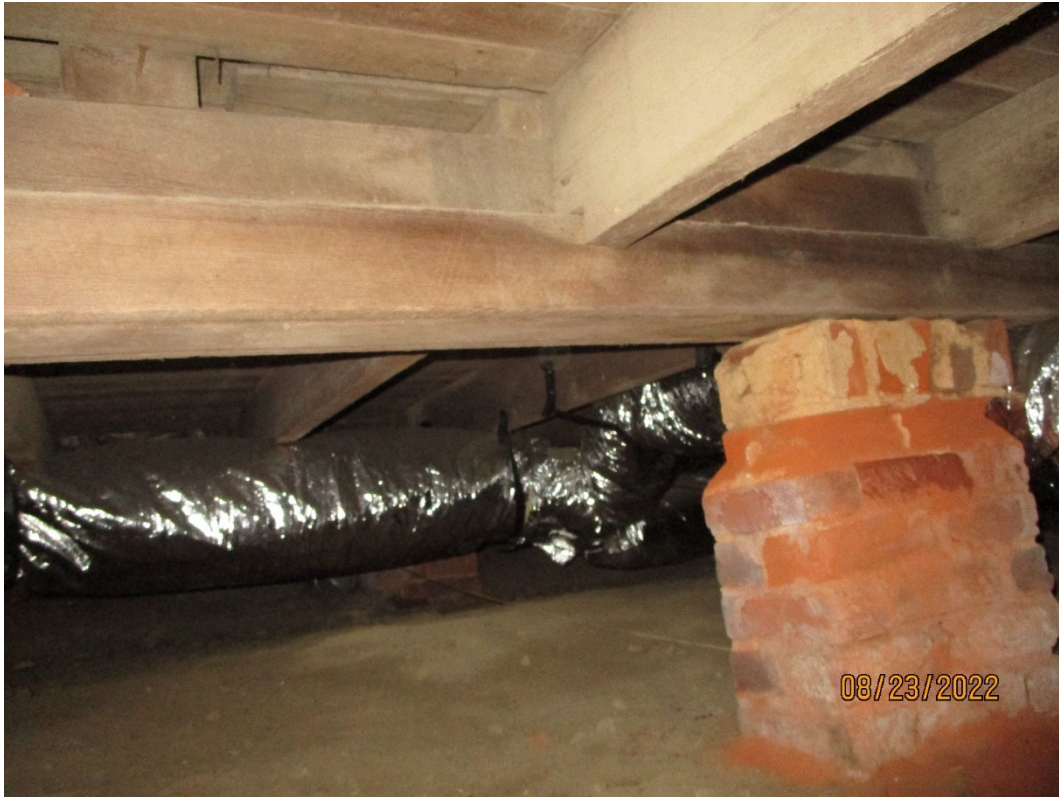
Crumbling Foundation(3) supporting hallway wall
