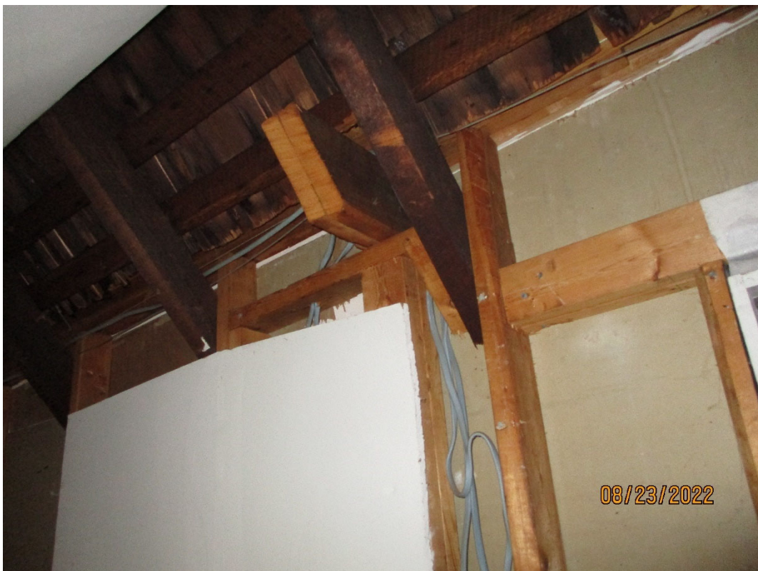
Original roof structure cut with no support
