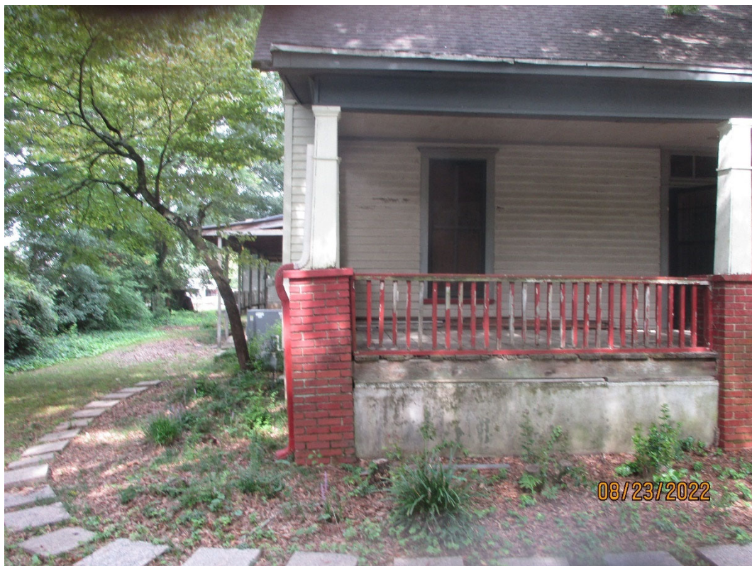
Front porch pilaster is out of plumb, column is rotting, infill wall is settled
