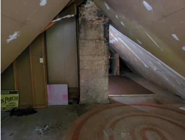
Figure 28 attic "bedroom" showing insufficient head height at access
