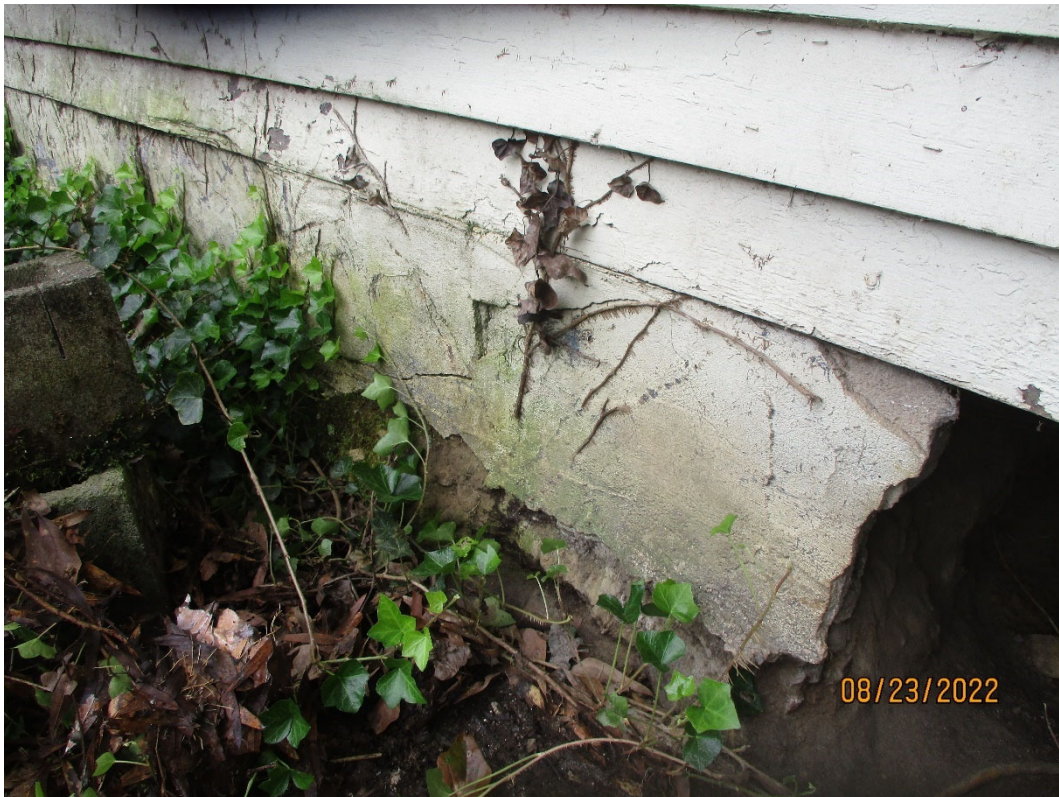
Undermined foundation wall on north side of property
