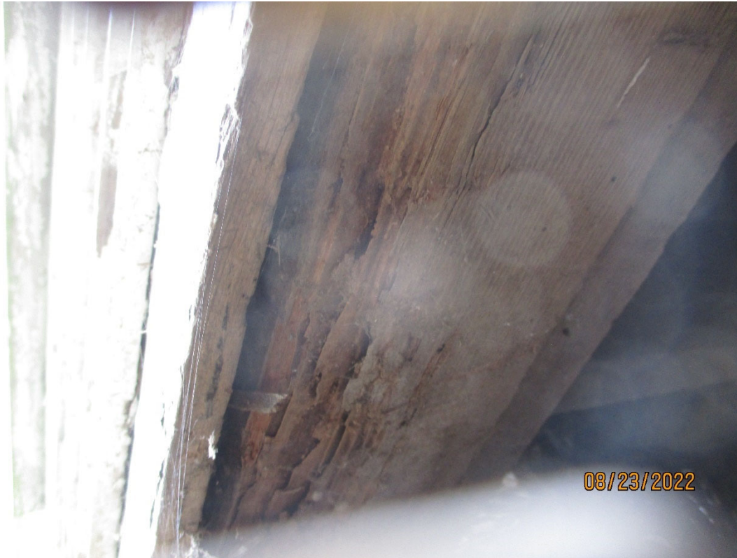
Insect damage on exterior sill beam below exterior wall.
