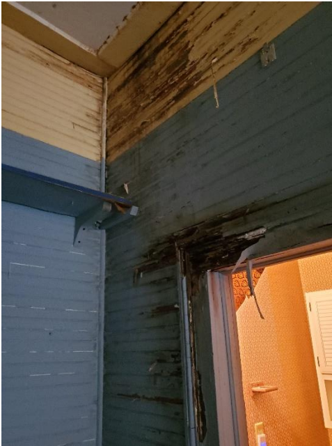
Figure 21 water damage in hall on wood board walls
