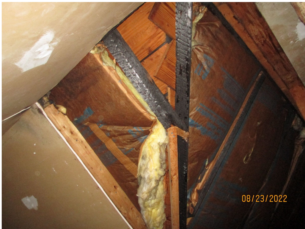
Fire damage observed in roof framing
