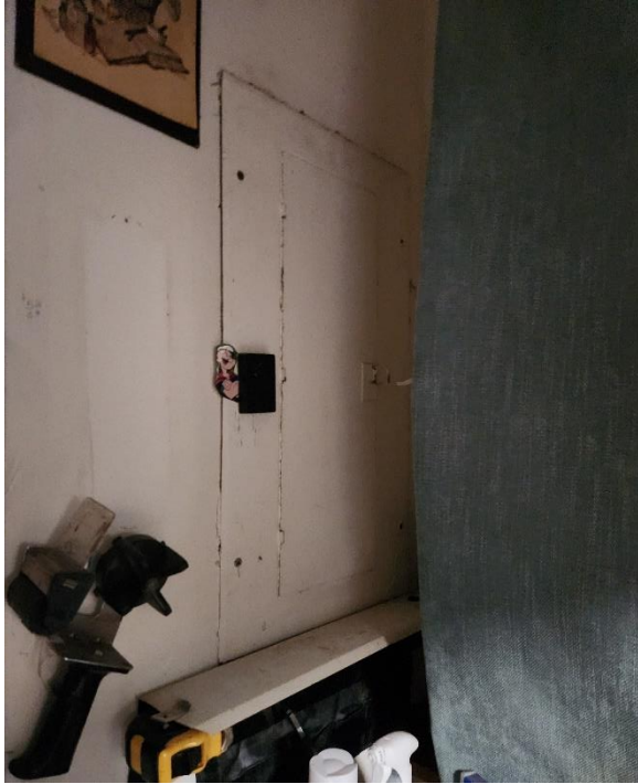
Figure 22 Fuse box is not code compliant
