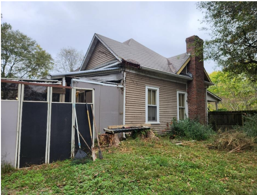
Figure 6 View of house from rear corner. Note reconstructed chimney and damaged rear eave, as well as non-historic exterior kitchen.
