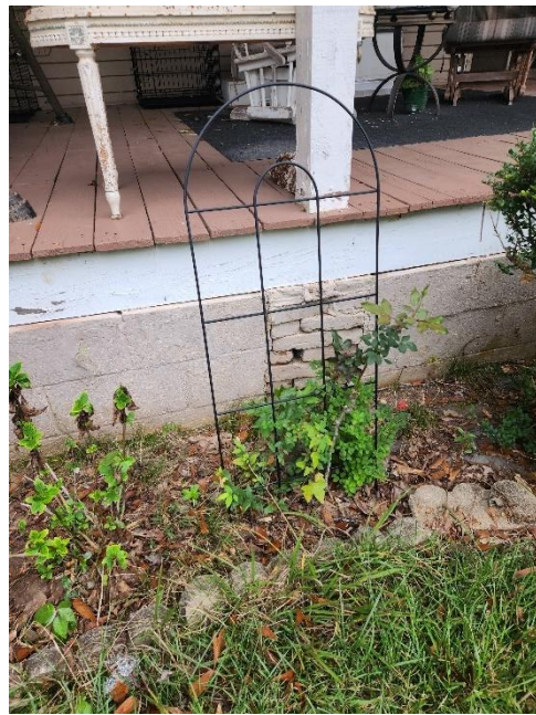
Figure 9 Foundation showing brick damage and concrete block infill
