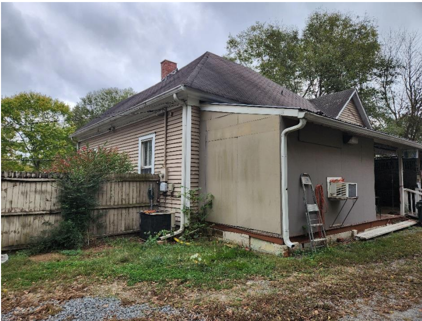
Figure 4 Rear of house showing filled in rear porch. Note deteriorated piers.
