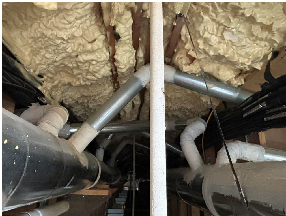
Attic duct work and foam insulation
